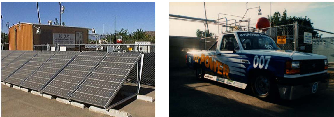
Figure 2. CE-CERT solar hydrogen research facility and hydrogen vehicle refueling station.
